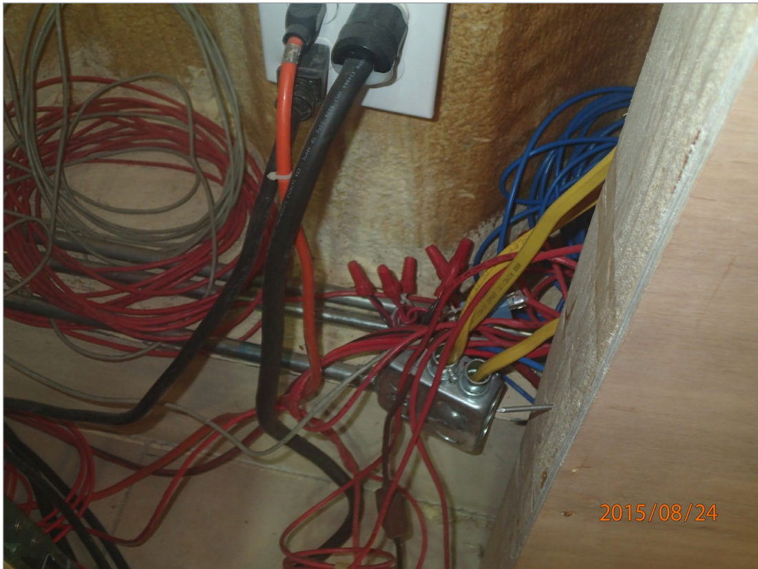
Figure 5. Missing junction box with exposed energized wires (Deficiency No. KAS-EL-150828-074) Source: DoD OIG, PO-TAD
