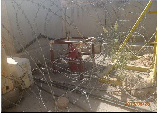
Figure 8A. Fire hydrant obstructed and inaccessible by concertina wire (Deficiency No. KAS-FP-150828-137) Source: DoD OIG, PO-TAD
