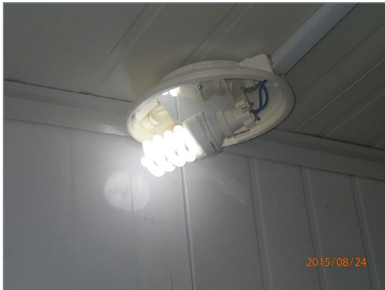
Figure 4. Light fixtures were missing lens covers and wiring was exposed (Deficiency No. KAS-EL-150828-076) Source: DoD OIG, PO-TAD
