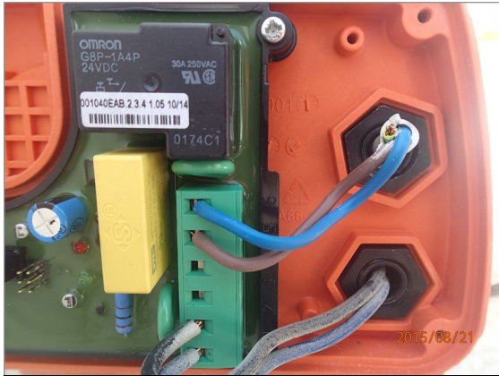
Figure 3. Water circulator motor with the ground conductor cut or missing (Deficiency No. KAS-EL-150828-023 Source: DoD OIG, PO-TAD
